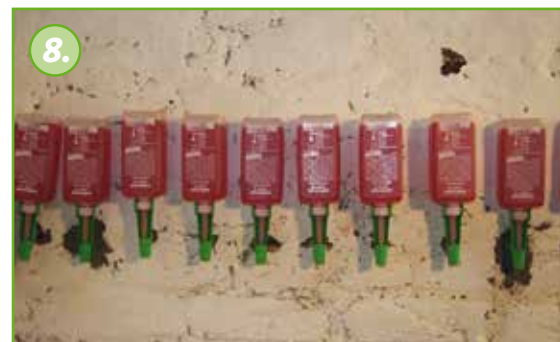
8. The pressureless injection of KÖSTER Crisin 76 Concentrate into the masonry starts immediately after the installation of the cartridges.
