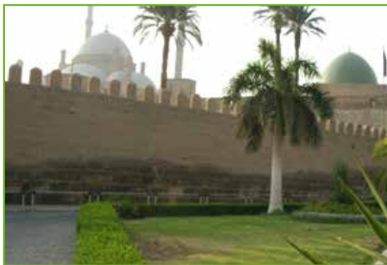
Example for rising damp
