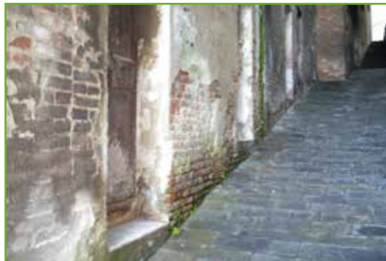
Destruction of render and mortar joints
