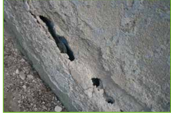
Damaged plaster / render
