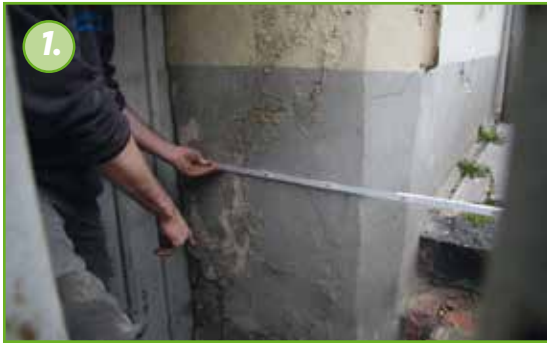
1. The masonry is from 1750, the existing plaster is damaged. The salt and moisture contents are high.
