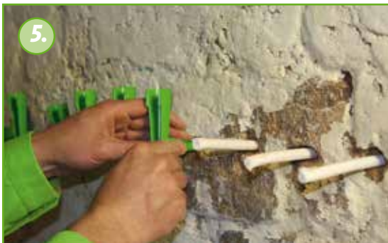
5. The KÖSTER Suction Angles are installed so that the KÖSTER Capillary Rods reach into the supply chamber of the KÖSTER Suction Angles.
