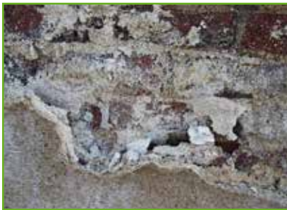
Typical damage through salt efflorescence.
